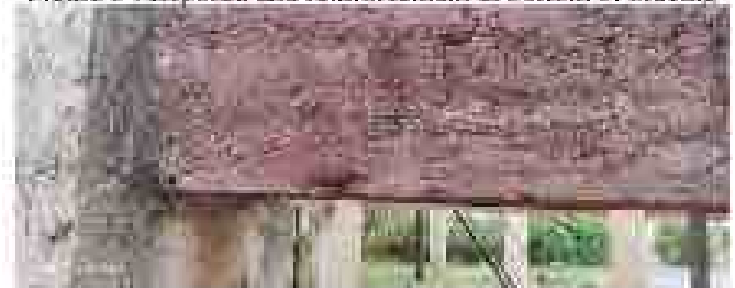
Figure 6: Cracks in bracing
