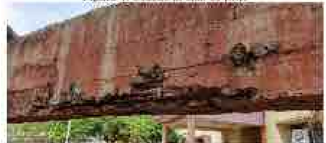
Figure 5: Exposed reinforcement at bottom of bracing
