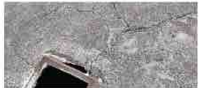
Figure 4: Cracks in slab of ESR
