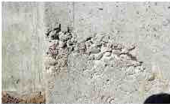
Fig.22 Honeycombing in concrete
